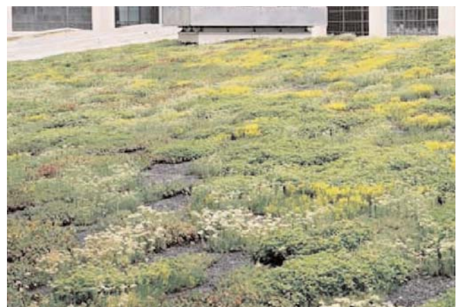
Photo 13 - Grown-on System 36 months after installation
