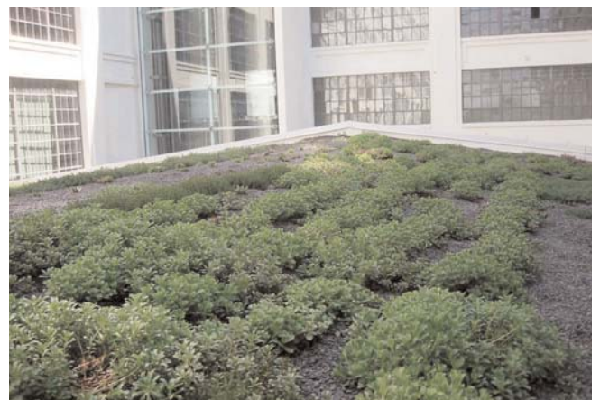
Photo 12 - Grown-on System 18 months after installation
